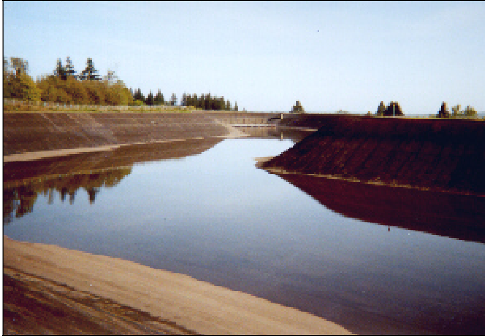
Photograph 1: Franzen Reservoir before the Rehabilitation Construction (Standing at the northwest end and looking southeast).
