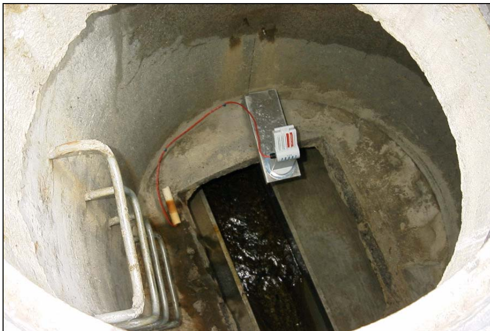
Photograph 3: Ultrasonic Level Sensor with Palmer-Bowlus Flume (Subdrain outlet manhole)
