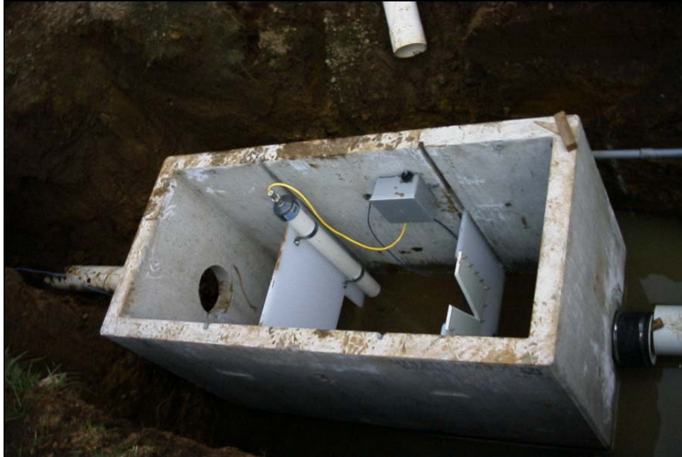
Photograph 2: Typical Weir Box for Monitoring Flows from the Seepage Collection Trenches (Weir 2 during installation including seepage collection piping entering and discharge piping exiting the weir box)
