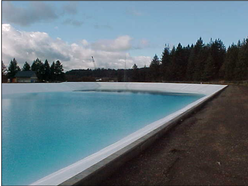
Photograph 4: Franzen Reservoir after the Rehabilitation Construction (Standing on the southeast cut slope looking northwest)
