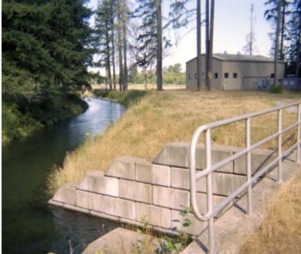
Geren Island Temperature and Flow Monitoring System Stayton, Oregon
